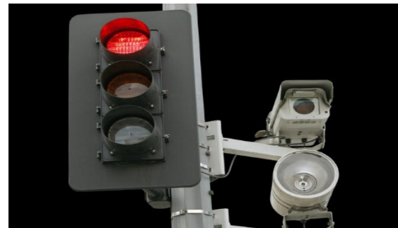
Figure 2: Cameras installed on red light.
